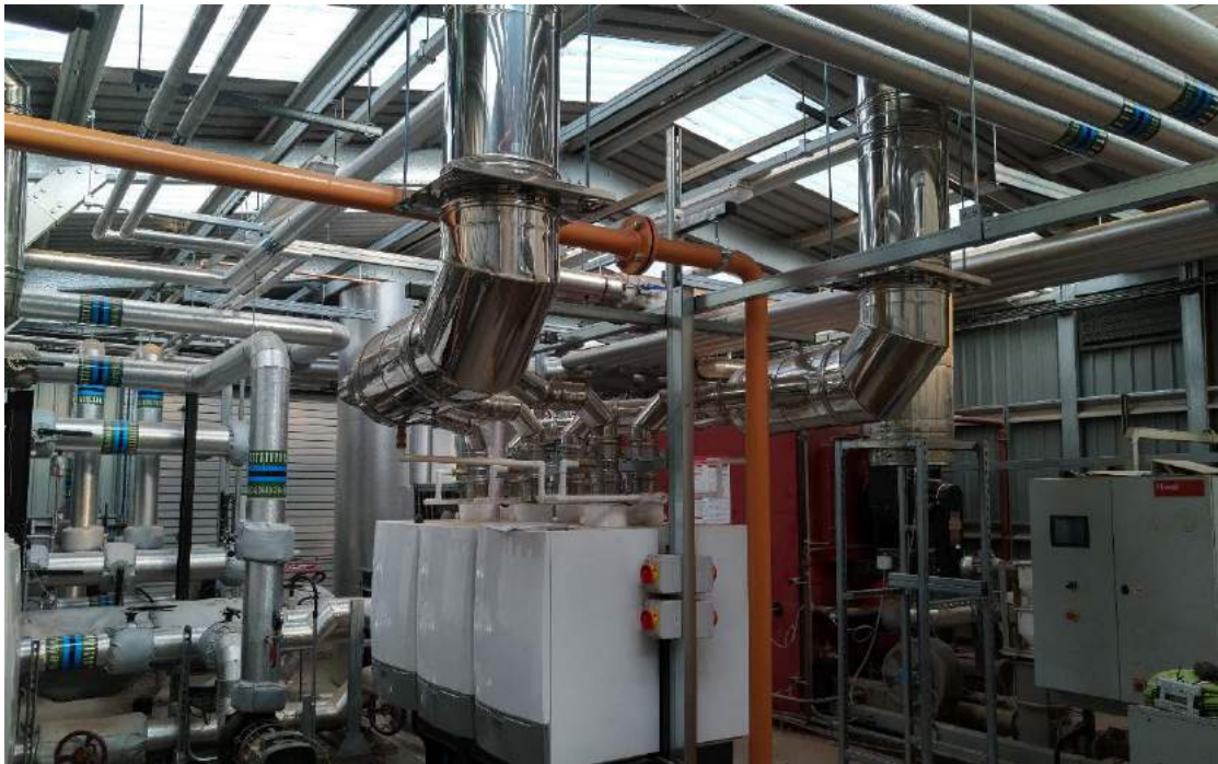
Inside the Combined Heating Plant at Brackenhurst Campus
